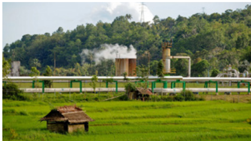
Asian Development Bank Lahendong geothermal power plant, Manado, Indonesia
